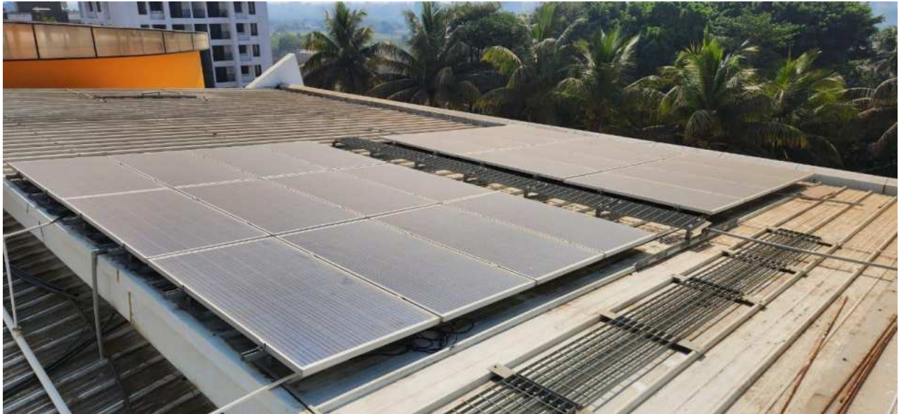
Plate 4: Solar panels in the premises
