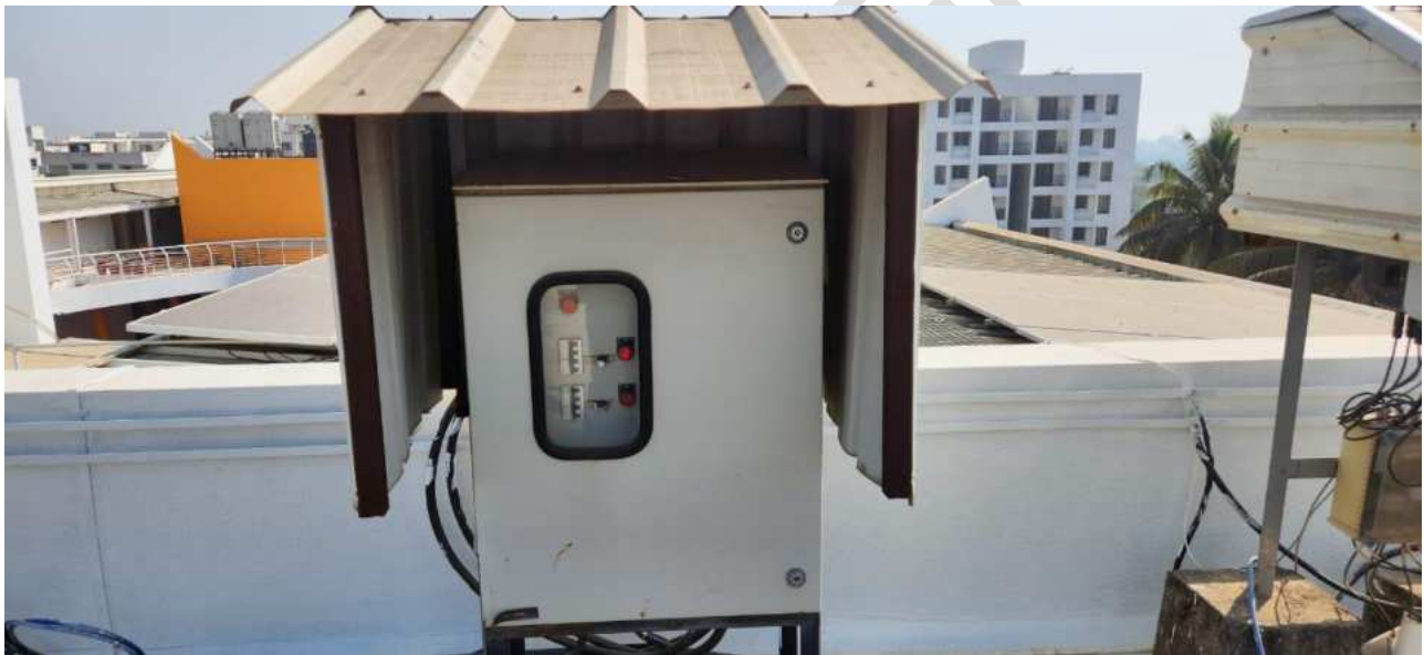
Plate 5: Solar inverter in the premises
